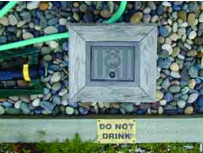
Exhibit 4.28 Green Operations Building: reclaimed water irrigation outlet
