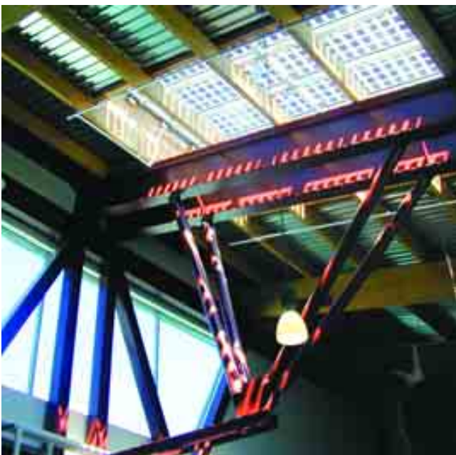
Exhibit 4.5 Works Yard: photovoltaic rooflight
