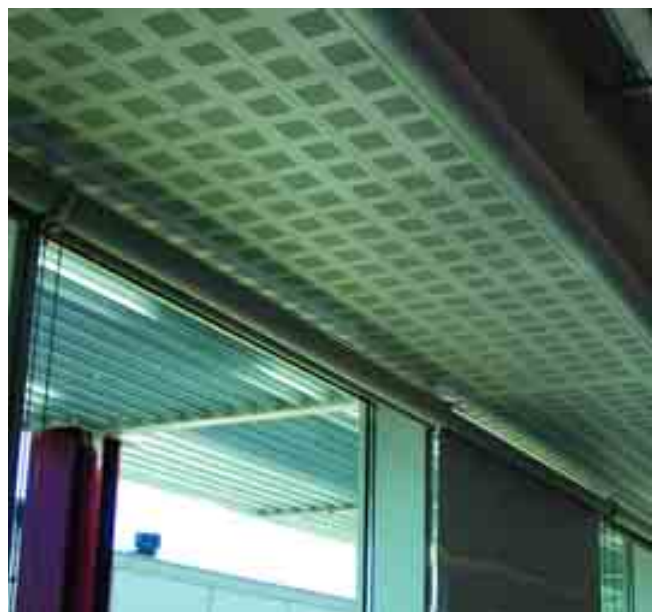
Exhibit 4.4 Works Yard: suspended radiant panels
